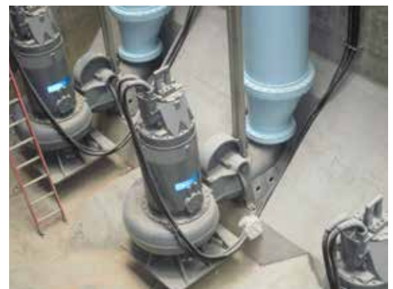
Pumps in the Sump
