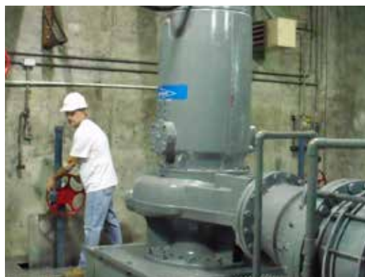
Lower level of Baltic Avenue pump station now housing one 135 HP and two 200 HP Flygt clog resistant dry pit submersibles pumps.
